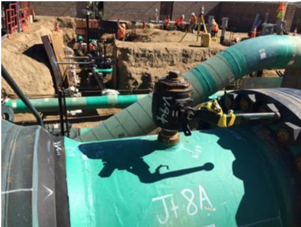
Figure 18: Large Valve Station with Numerous Above-Ground Features
