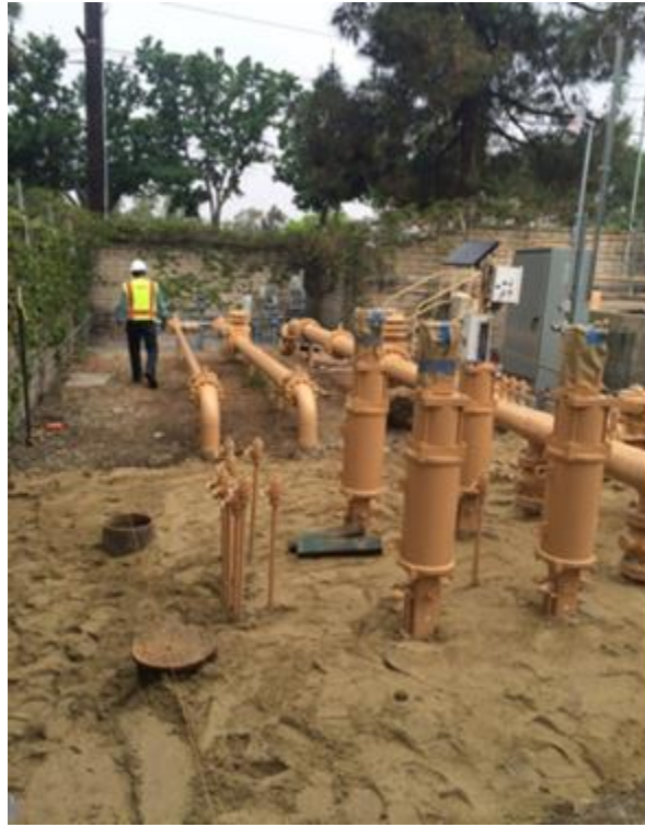
Figure 17: Above-Ground Valve Equipment
