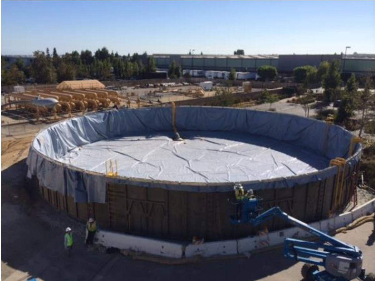
Figure 9: Lake Tank used for storing hydrotest water
