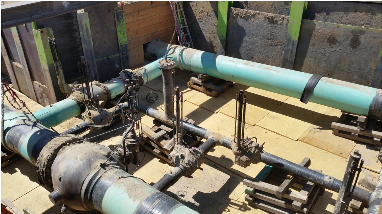
Figure 2: Existing 30" MLV 2002-6.81-0 and 20" Crossover valve 2002-6.81-2 prior to replacement. Blowdown valves are also shown. This large assembly was replaced and the newly installed 30" MLV, and 20" and 16" Crossover valves were automated.
