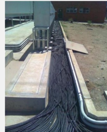
Hard wired substation
