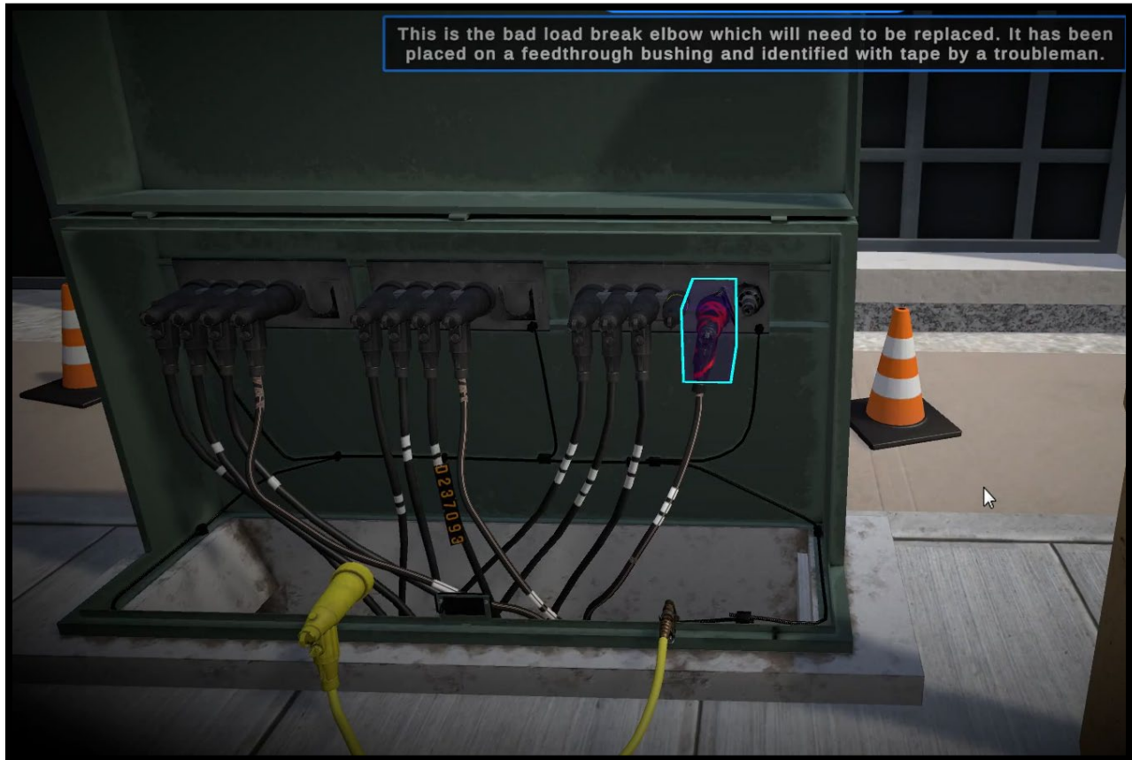
Figure 2: Faulty Load Break Elbow
