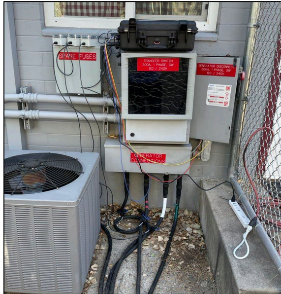
Figure 5-6. MBESS Connected to the Permanent Connection Box at Pine Valley CRC
