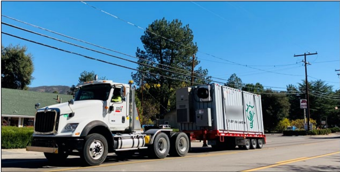
Figure 5-13. Photo of MBESS on the Road during Transportation from CRC 1 to CRC 2
