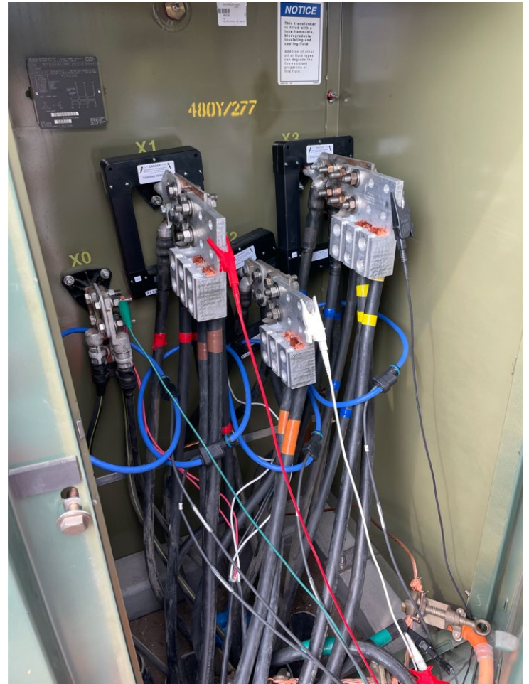
Figure 2: MBESS Connection to MGBW Transformer
