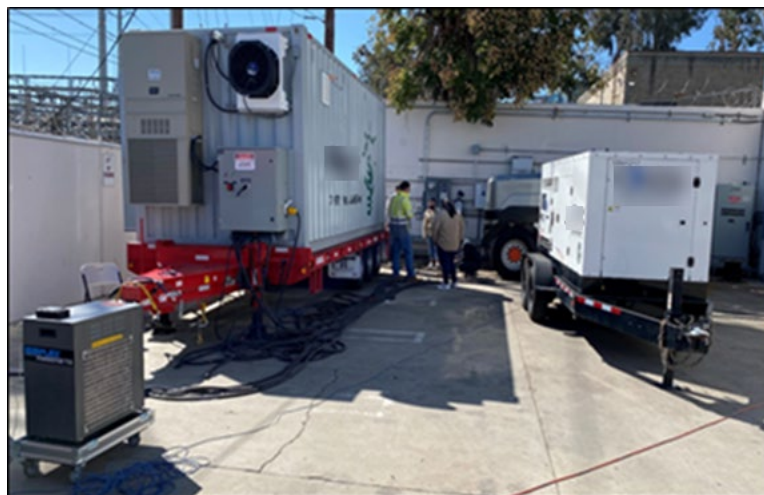
Figure 5-9. Photo of the MBESS at ITF during the SAT
