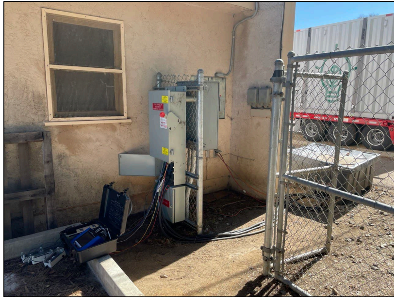
Figure 5-4. MBESS Connected to the Permanent Connection Box at Dulzura CRC
