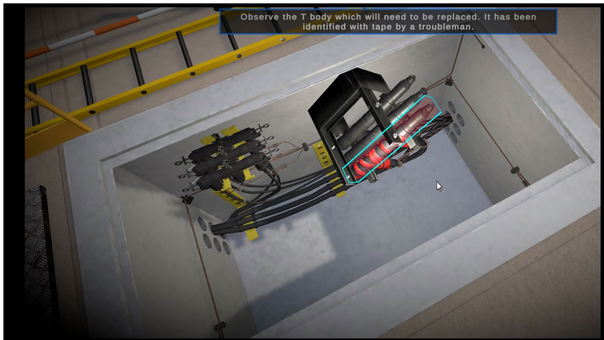
Figure 4: Failed 600-AMP T Connector
