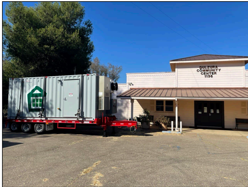
Figure 5-3. Picture of the MBESS in Front of the Dulzura CRC for Demonstration 1
