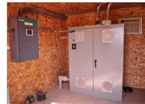
200 HP MOTOR STARTING VFD & 100 HP REGENERATION VFD WITH LOCAL CONTROL PANEL.
