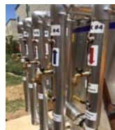
Solar thermal heat exchanger piping
