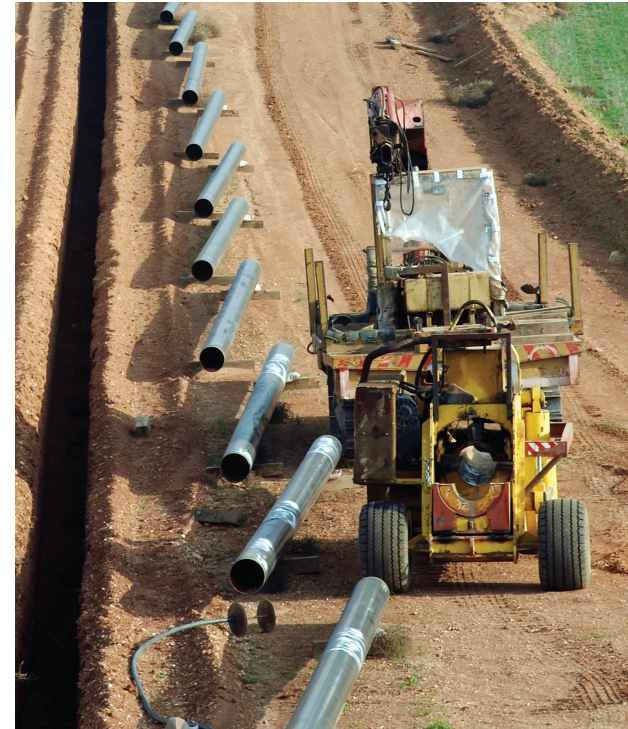
Natural gas pipeline sections are arranged along a trench before being welded together.
